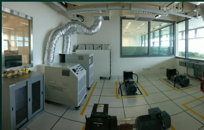
Electric Power and Intelligent Control (EPIC)
